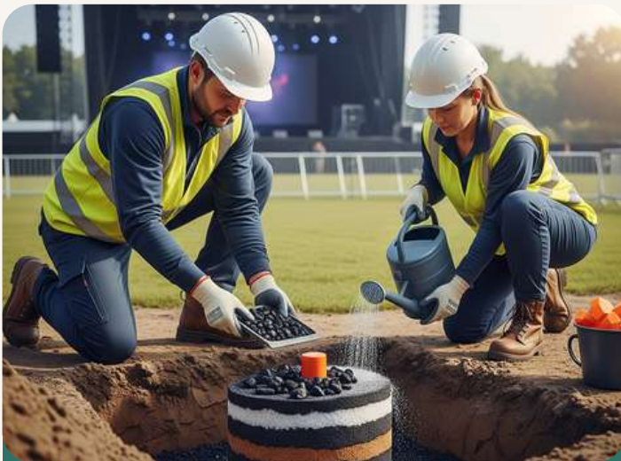
Use Soil Enhancers & Watering method: Improves earth resistance and activates layers to aid conductivity
